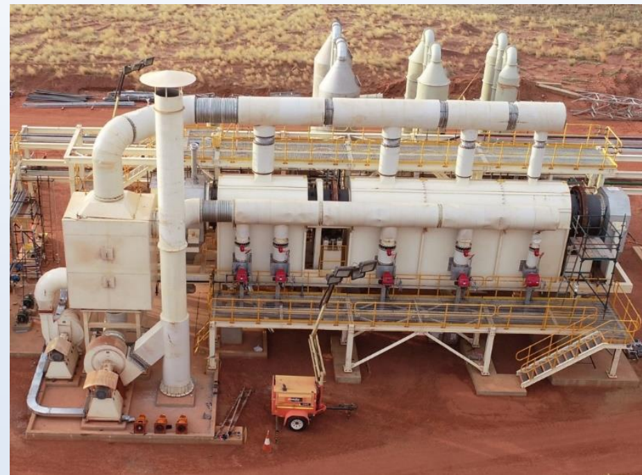
Indirectly heated kiln at Browns Range Pilot Plant
